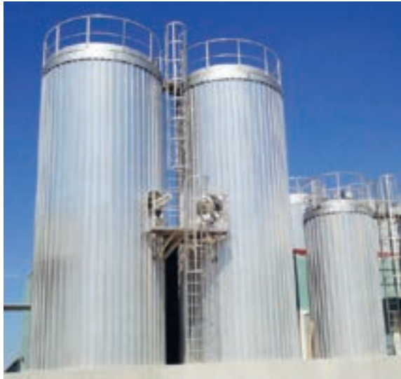
stainless steel tanks
